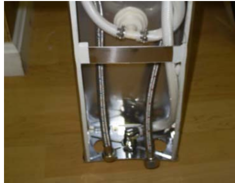
Cold & Hot Pipes
