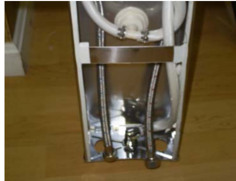
Cold & Hot Pipes
